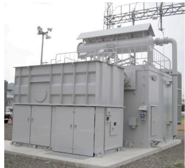
66kV 50Mvar Shunt Reactor
