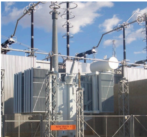
800/√3kV 438/3Mvar Shunt Reactor
