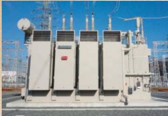
● 450MVA transformer for Higashi-Osaka substation
