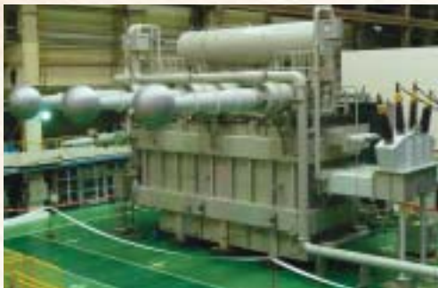
● Factory test of 300MVA transformer for Minami-Himeji substation
