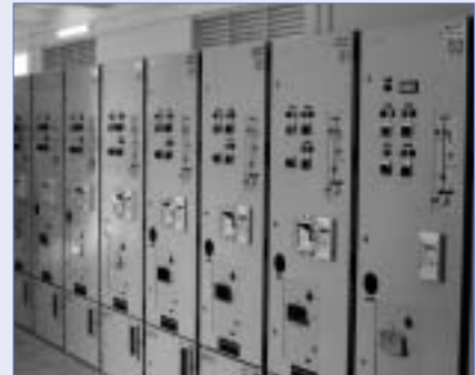
24kV dry air-insulated C-GIS
