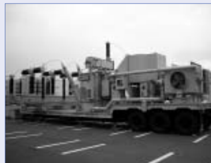
132kV mobile substation
