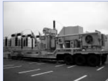
132kV mobile substation
