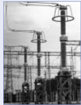
266kV polymer insulator type lightning arrester
